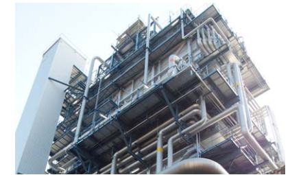
■ The highly efficient naphtha cracker at the Tokuyama Complex
